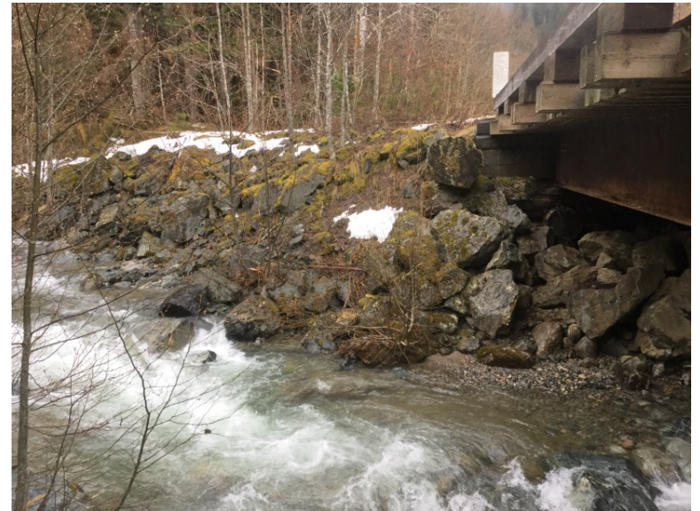
Upstream left bank riprap failure
